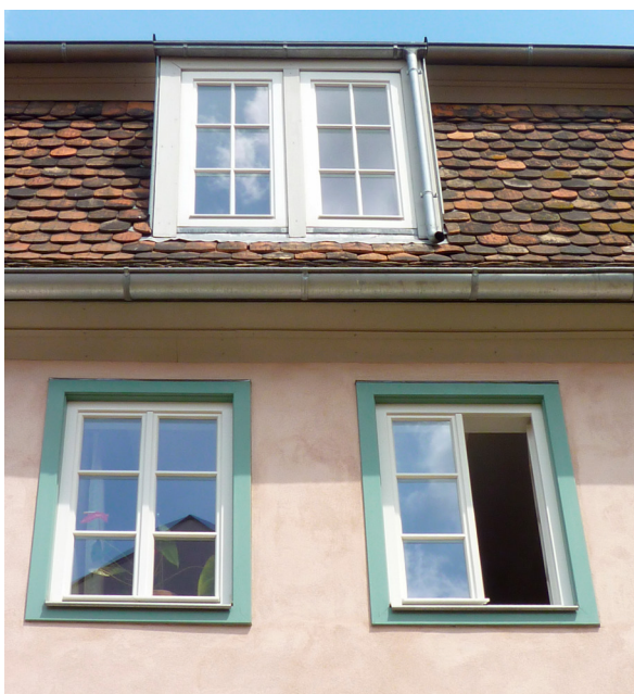
05 and 05a 260 year old half-timbered house with earth infill and internal insulation
