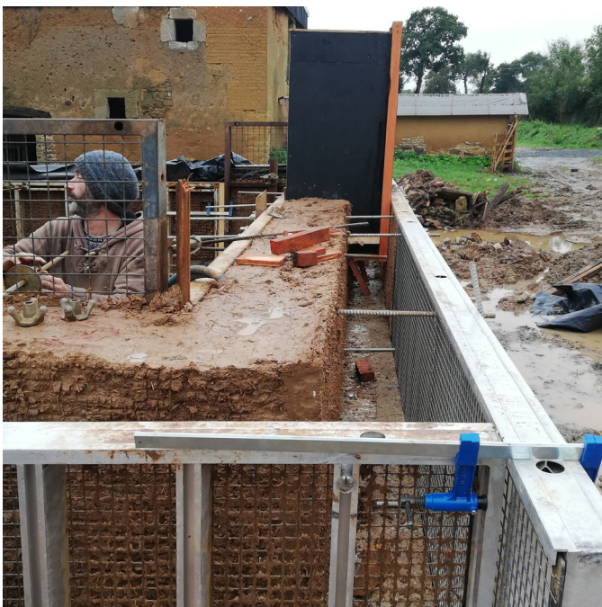
10 Completed first lift of cob with formwork shifted outwards to receive hemp shives
