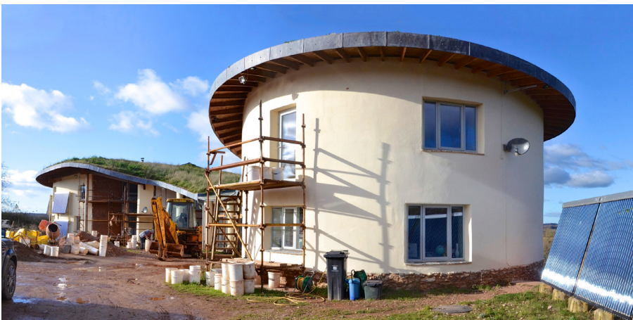
03 Zero carbon cob house build by Kevin McCabe in south Devon (UK)
