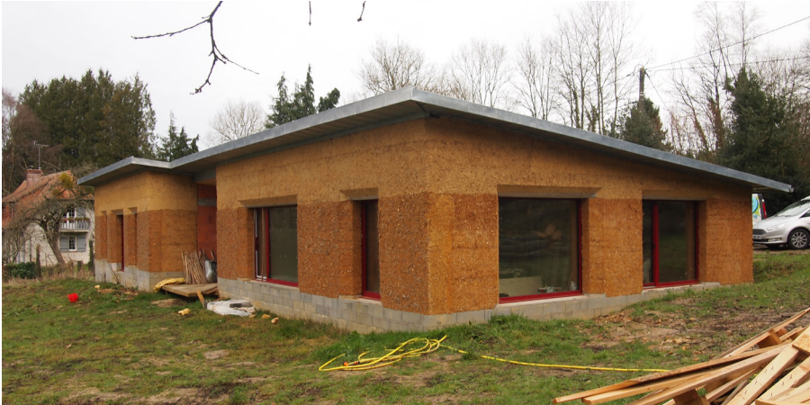
02 Cob dwelling in Normandy by Les Frères Bon, with composite walls made of two layers of shuttered cob with cork shiv insulation in between
