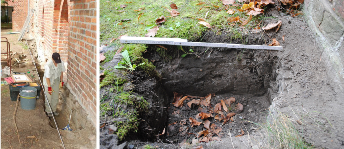
02 Retroactive masonry waterproofing at the Heilige Geist Church, Teupitz (13th/14th century). A vertical barrier was inserted in 2008 using local glacial till (left photo, by T. Wondoll). The density of the waterproofing layer was checked in 2014 and found to be functional (Michette 2015) (right photo).
