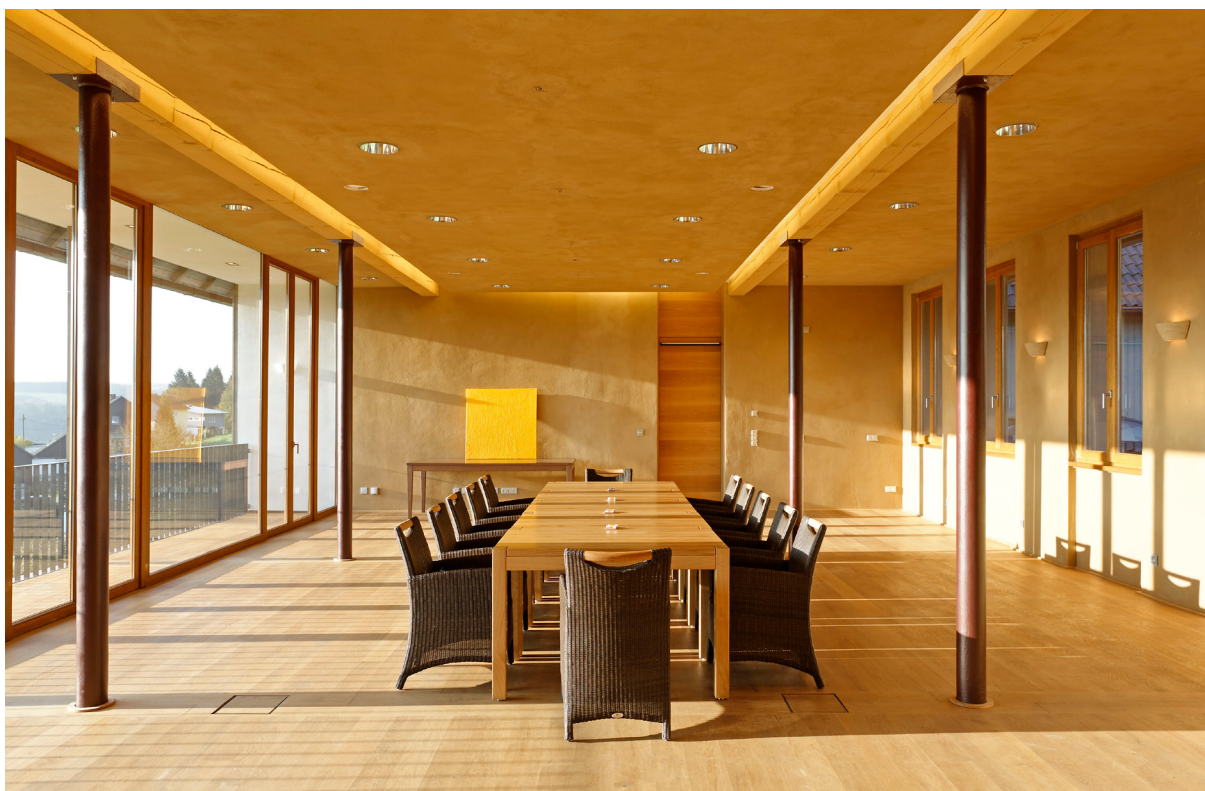
11 Climate panel ceiling for heating and cooling in a conference room at EcoLut Lehmhaus in Engelskirchen, Germany
