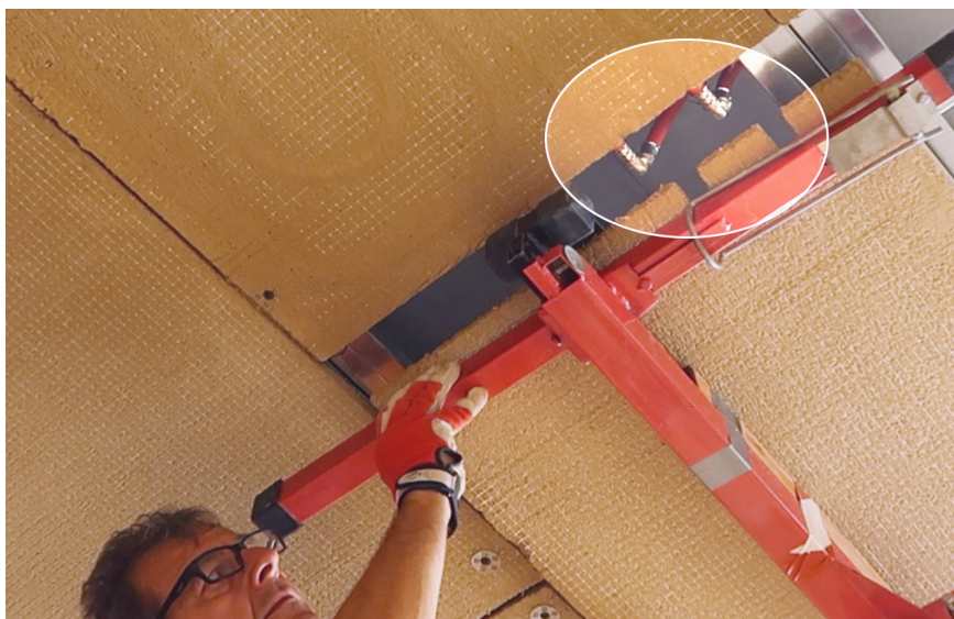
06 Pre-cut earth panels accommodate the pipe connections of the adjacent WEM climate panel to provide a flat, continuous surface for subsequent plastering
