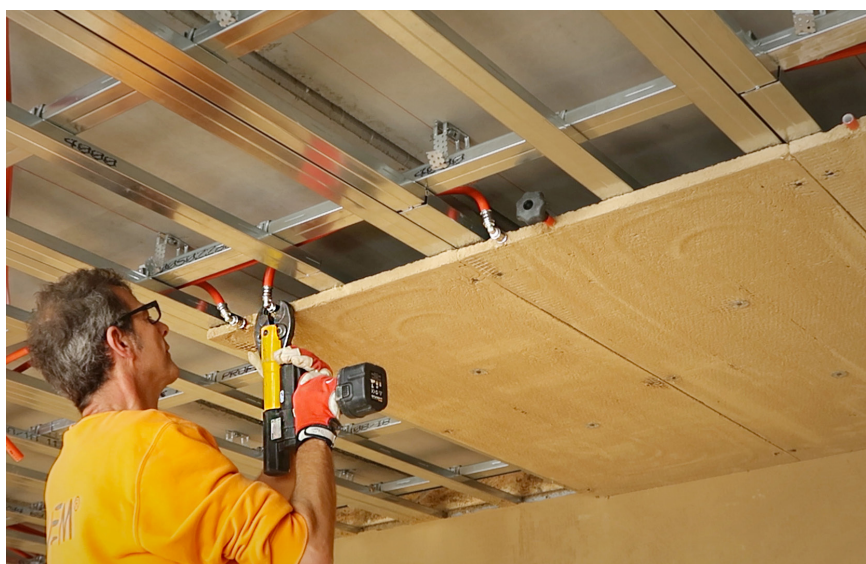
07 The climate panel elements are screwed to the suspended ceiling and the pipes linked together via compression-fitted connecting pieces
