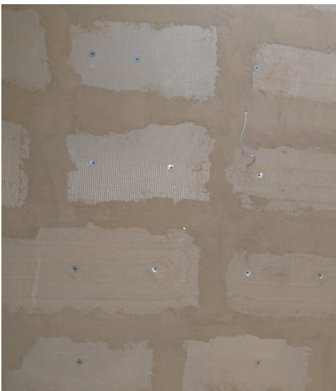
04 WEM climate panel ceiling after installation and joint filler at Dr Kauer vineyard
