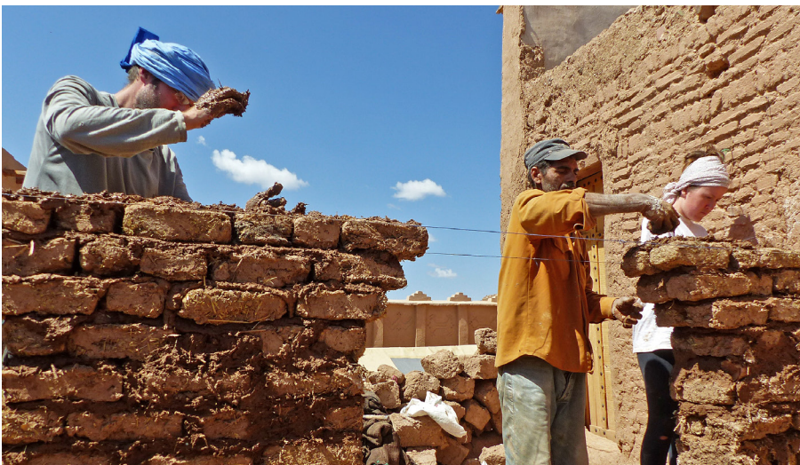
01 Building the wall of an arcade passage on the roof of the Kasbah des Caïds, Morocco
