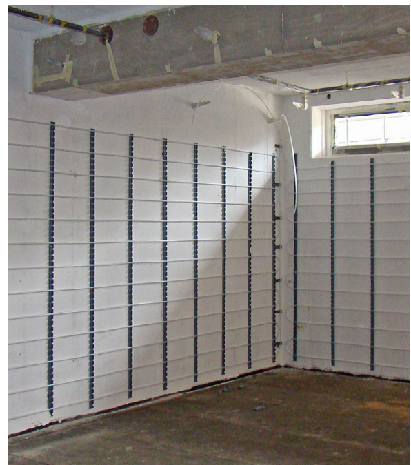
04 Pipes of the wall heating registers prior to application of the clay plaster
