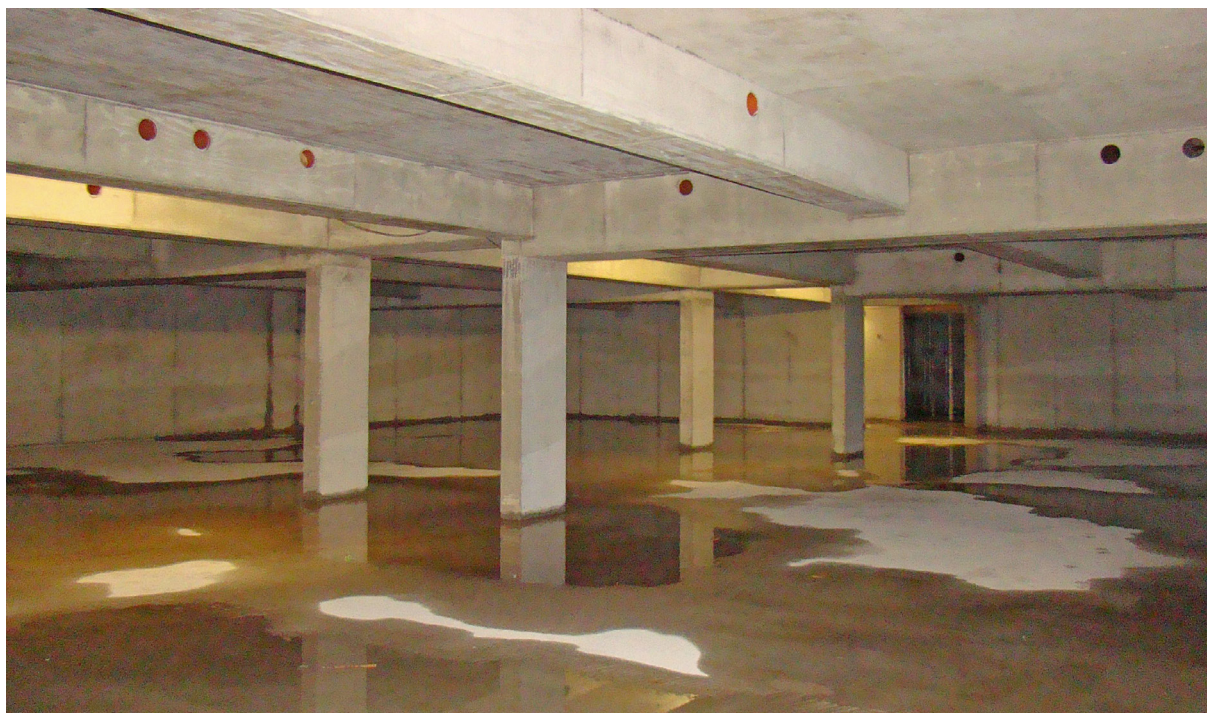
10 Depot D113 during the construction phase showing rainwater pooling on the ground
